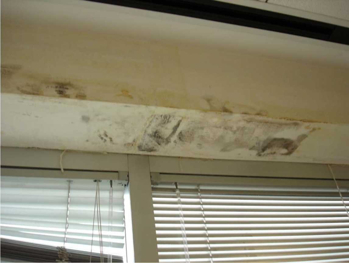
Fungal growth under vinyl wall paper above window in WBOB October-2005
