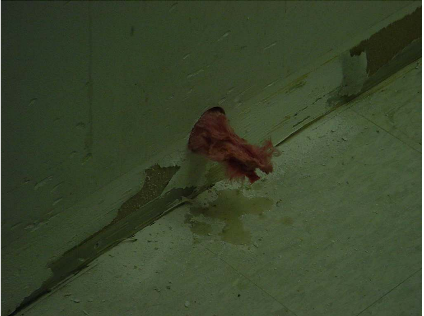
Wet insulation in water damaged wall 48 hours after flood.
