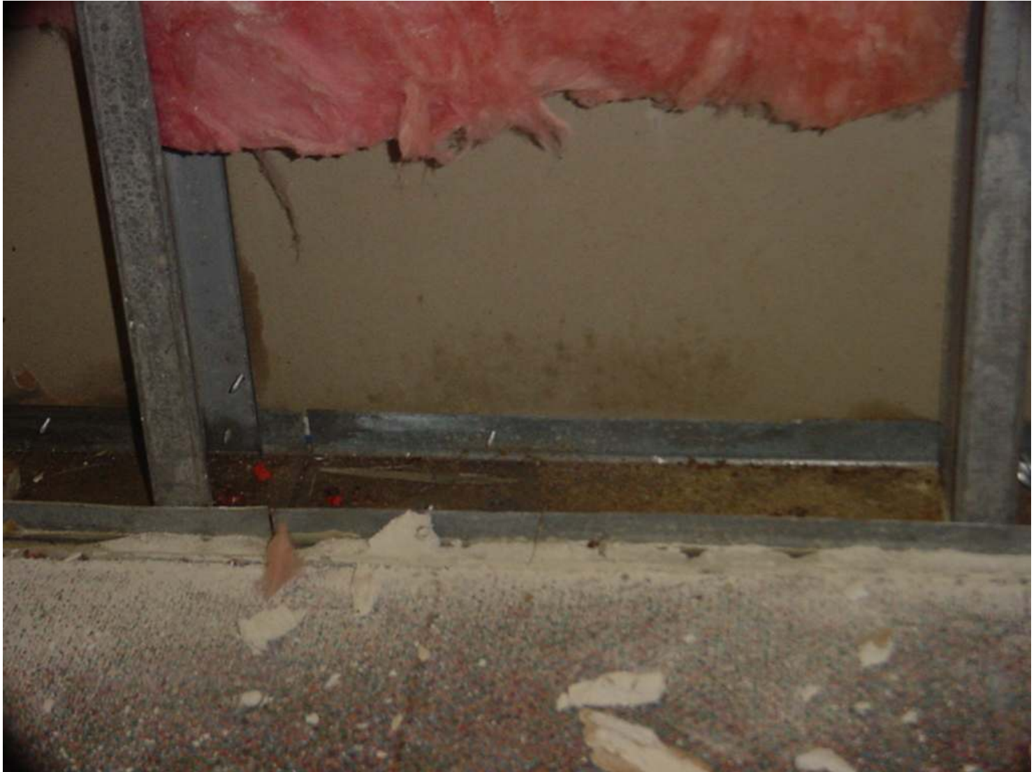
Mold growth less than 60 hours post flood
