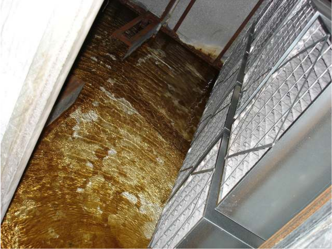
Standing water inside air handling unit – April, 2006
