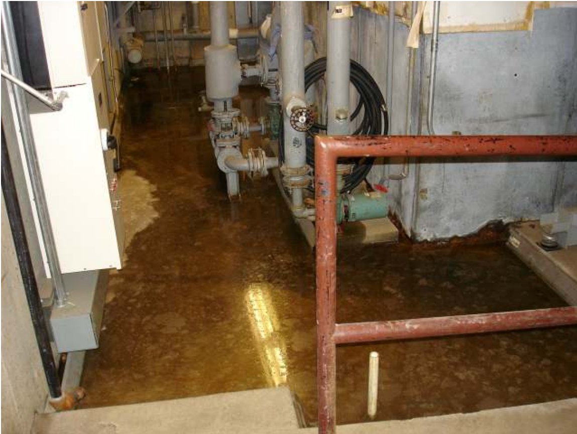
Williamson Hall flooded floor of mechanical space - April, 2006
