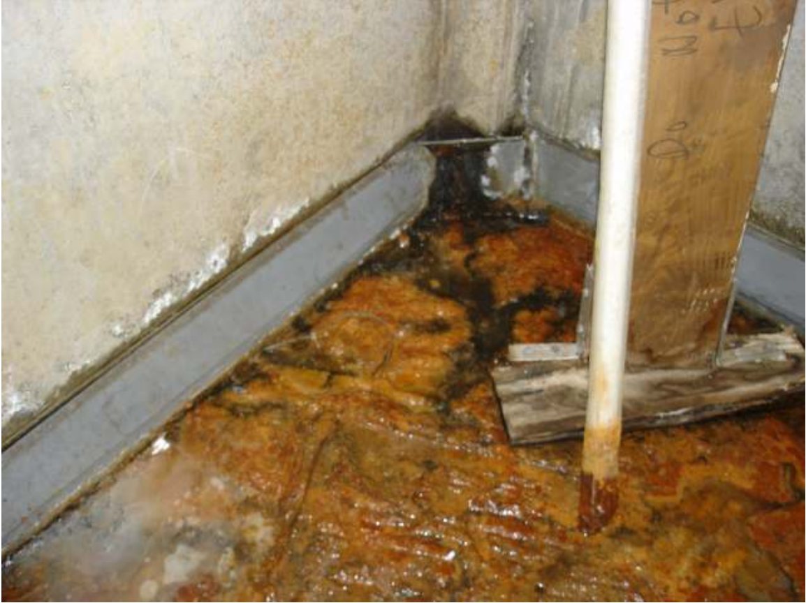
Slime on floor adjacent to ineffective perimeter drain system – April, 2006
