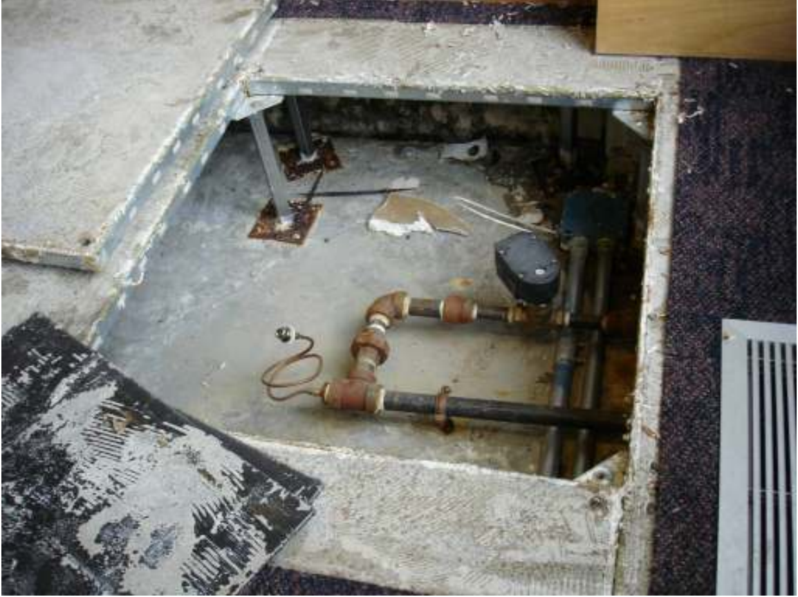
Rusting floor supports and mold growth below raised floor on sheetrock
