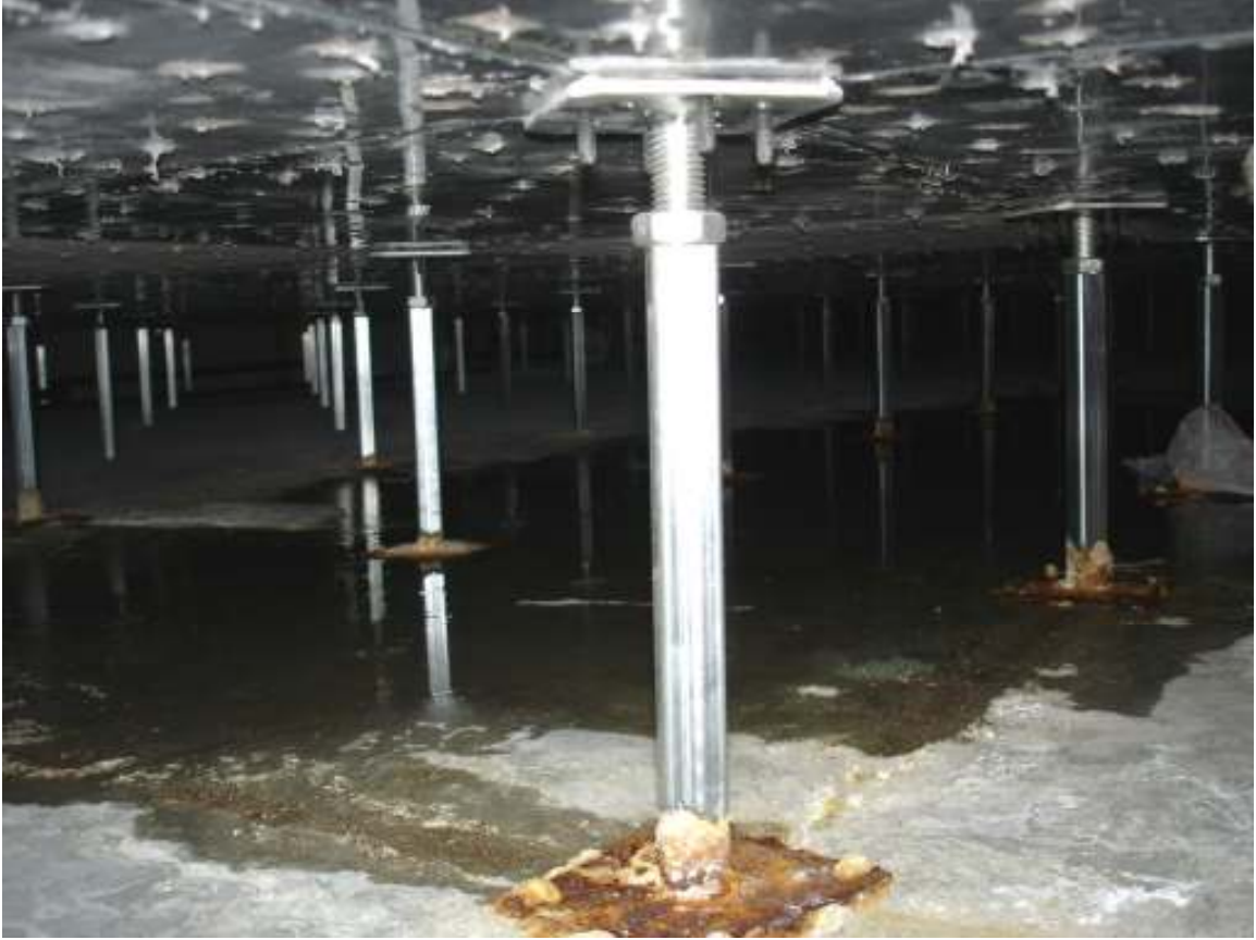
Standing water beneath floor
