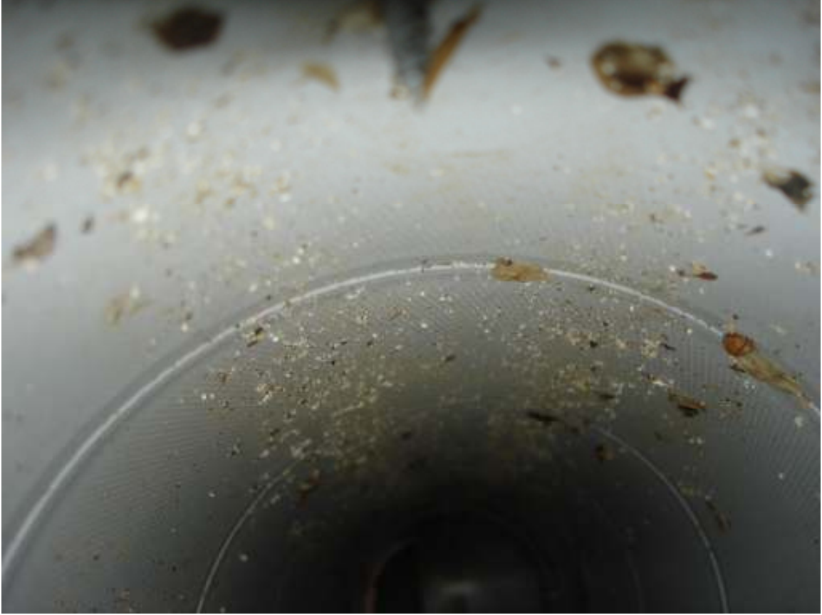
Debris on top edge of duct after filling with water – August 2006
