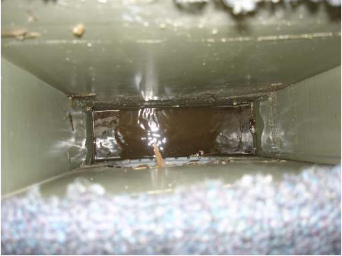
Sub slab ventilation ducts with standing water University Childcare center August, 2006
