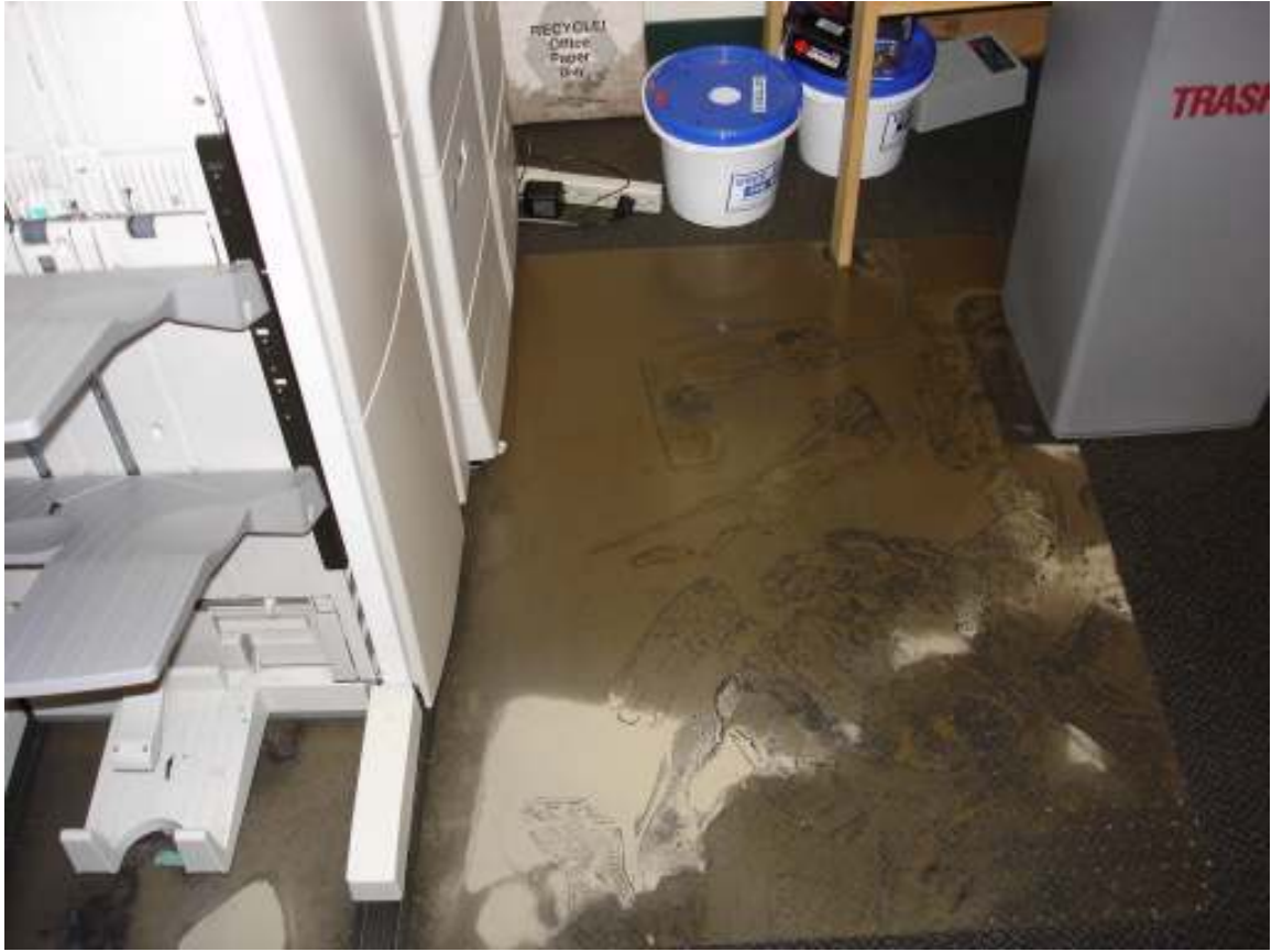
Mud and water discharged from below grade duct at University Childcare center August, 2006.
